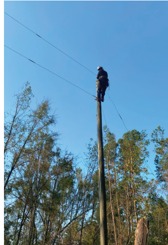
The water-logged ground was often too soft for bucket trucks, forcing ECE Apprentice Lineman Tate Peters to do a lot of climbing.
