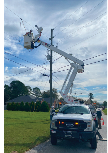
ECE Lineman Easton Soucy helping a neighborhood in Georgia get power restored weeks after it went out.
