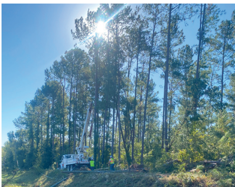
BELOW: Photo shows the height of the pines with an extended digger truck and linemen for perspective.
