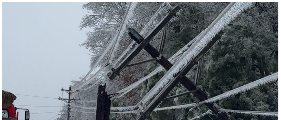
Photo courtesy Tallahatchie Valley Electric Power Association, showing ice accumulation and power line damage in the immediate aftermath of Winter Storm Fern.
